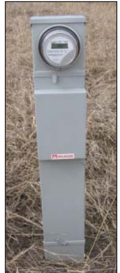
Figure 1-17a. Factory built meter pedestal example.
