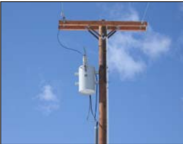
Figure 1-1. Pole with transformer.
