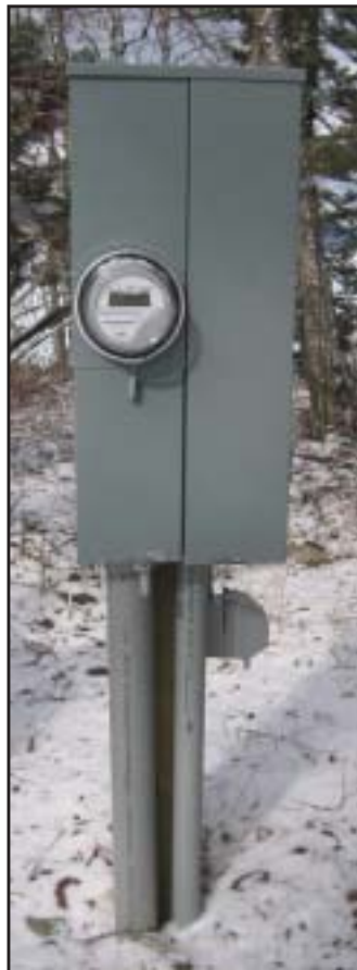
Figure 1-16a. Custom built meter pedestal example.
